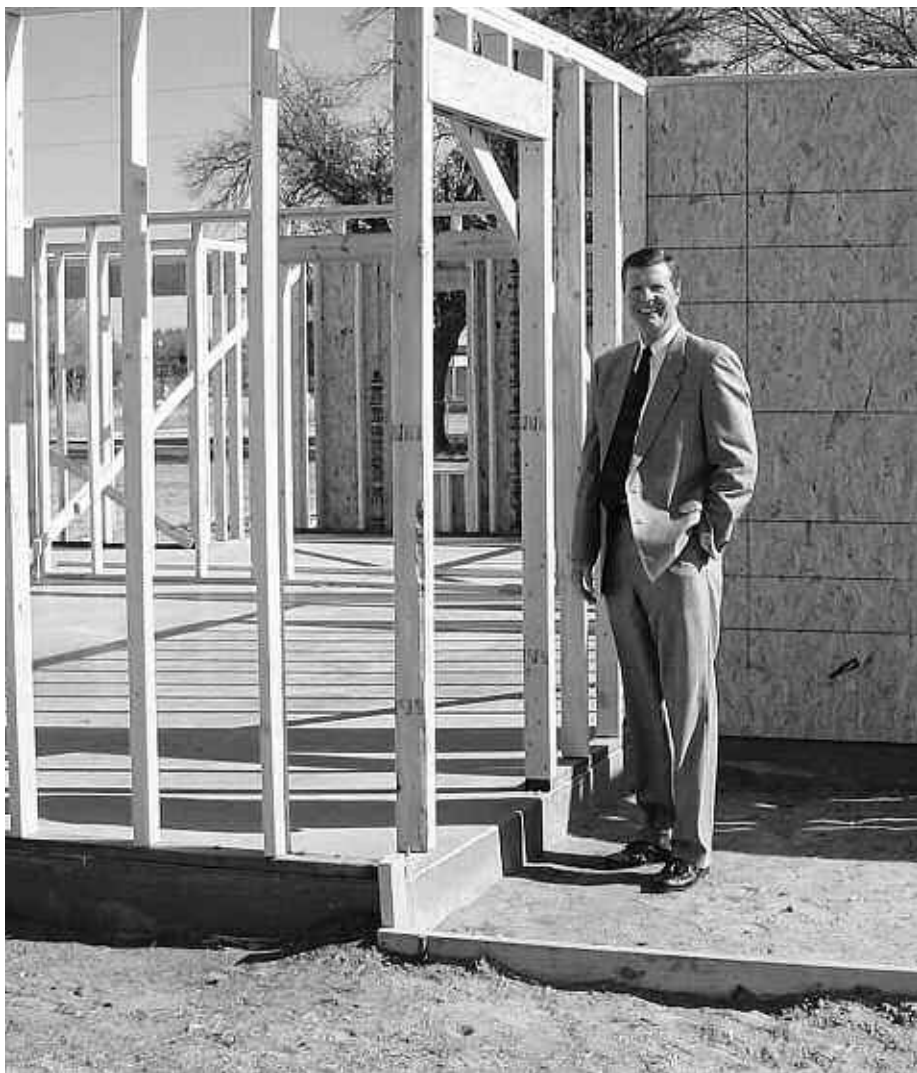
T.J. Parks, Superintendent of Tatum Schools, one of the pilot districts in the Rural Revitalization Initiative, stands in front of the house his students are building.
